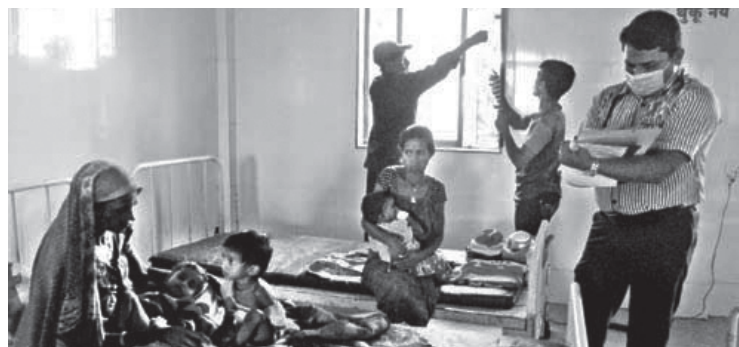
Children are exposed to infections as workers install grills at the windows. The children were not moved during the entire process.
